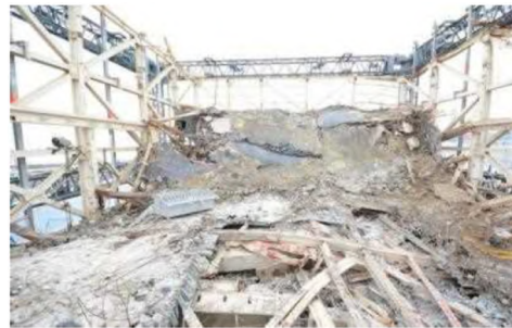
Condition of the collapsed south-side roof
